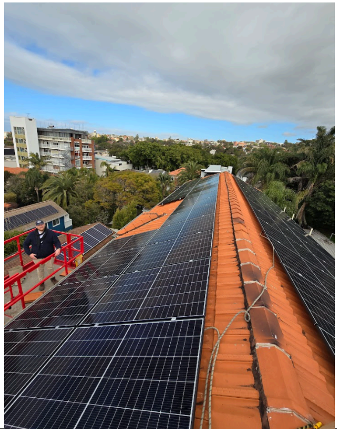
Figure 1. Solar panels installed at 31 Roscoe Street
